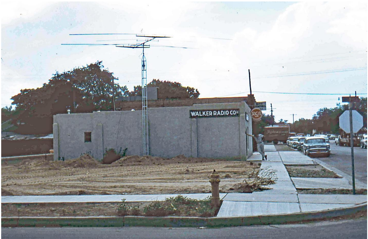
The parking lot getting paved in July 1958; note Len's ham radio antenna
